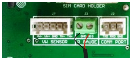
Figure 3-8: Connecting Rain Gauge cable
